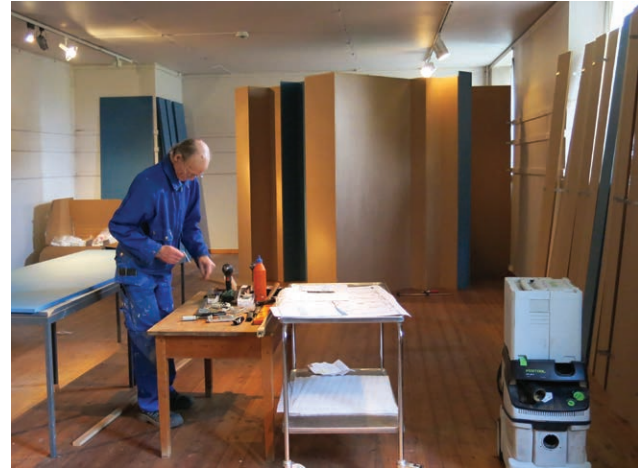
▼ Fig. 9: A small section of the wall system mounted on the 18 th of September 2015.
